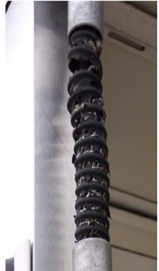
Deterioration of Stage II Connection hose, courtesy of VA DEQ Piedmont Office.
